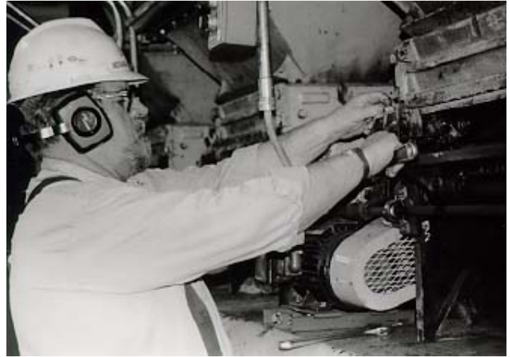
Utilities Equipment Operator Fred Norman inspects a boiler stoker at the Central Heating Plant. Unneeded parts from Ford Motor company's plant will be used for repairs as equipment is needed.
